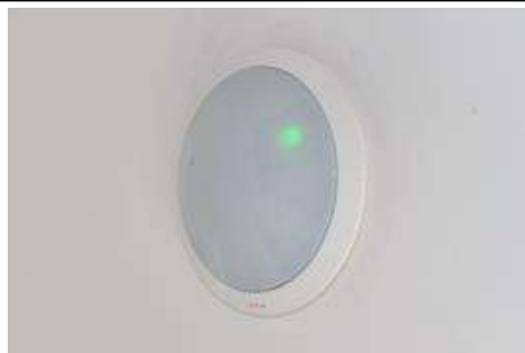
Figure 19: Emergency lighting unit
