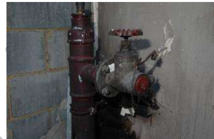
Figure 13: Fire mains outlet
