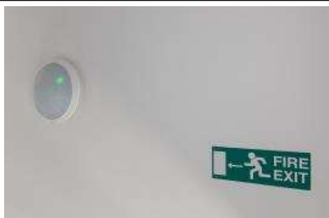
Figure 18: Emergency lighting unit
