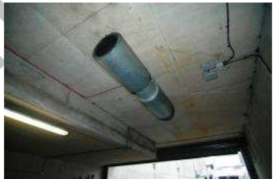
Figure 28: Smoke control system
