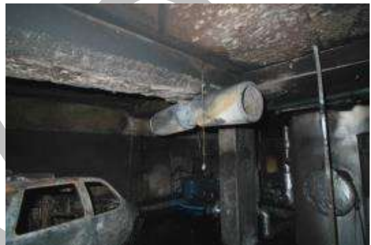
Figure 27: Smoke control system
