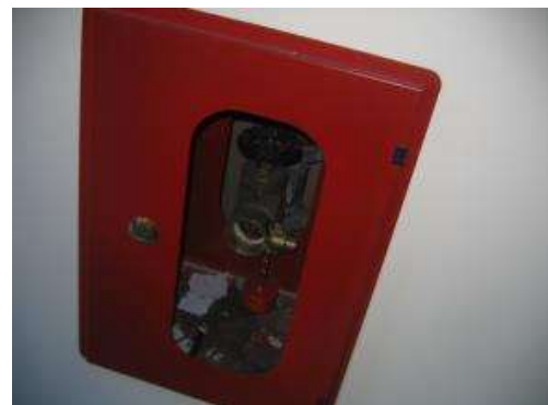
Figure 15: Dry riser landing valve
