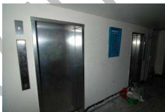
Figure 16: Firefighting lift and controls
