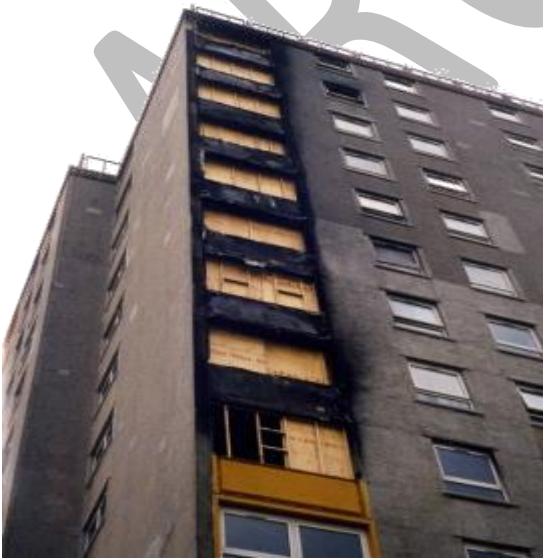
Figure 5: Post-fire damage illustrating the result of the Coandă effect
