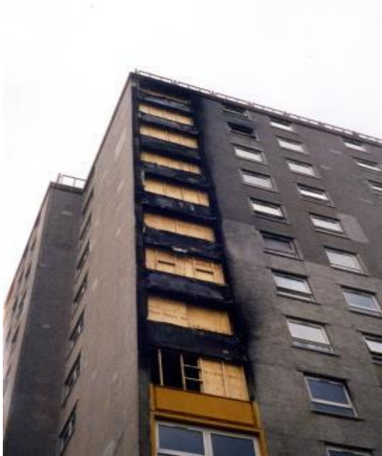
Figure 5: Post-fire damage illustrating the result of the Coandă effect
