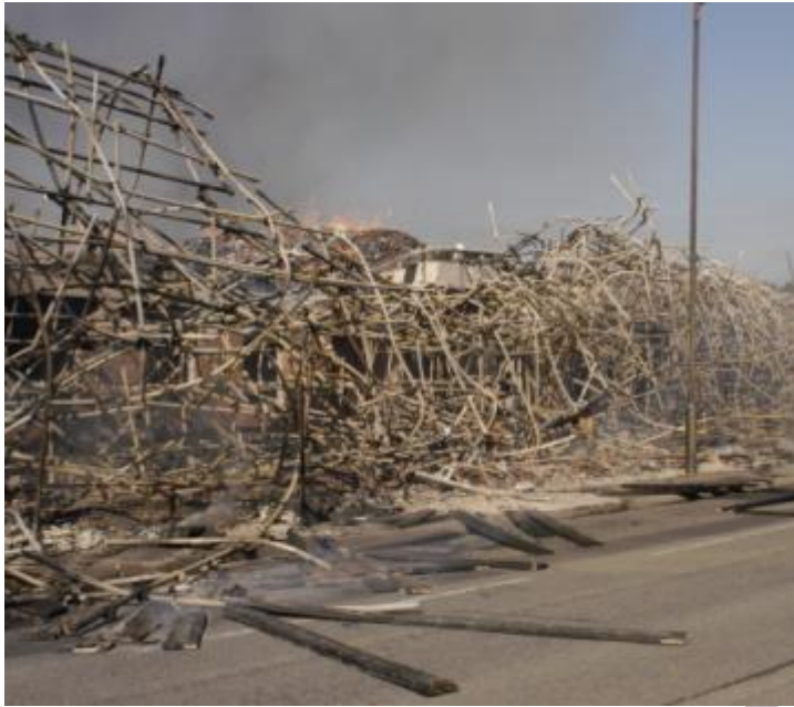
Figure 6: Post-fire incident site showing debris outside of site boundary – photograph courtesy of London Fire Brigade
