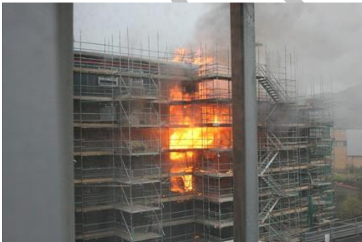
Figure 13: Scaffolding involved in a fire – photograph courtesy of John Dickie
