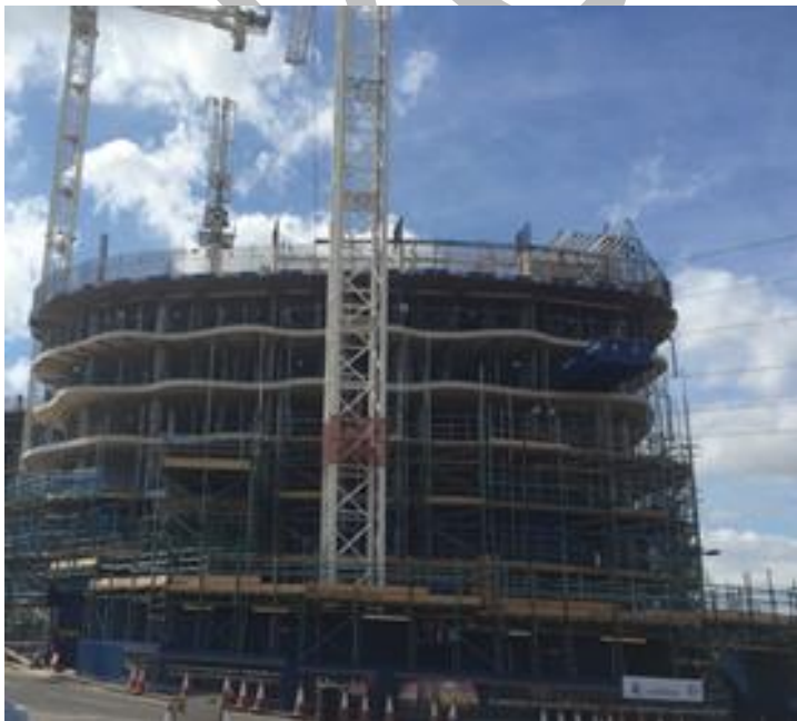
Figure 2: Building under construction showing cranes and scaffolding – photograph courtesy of Brian Massie
