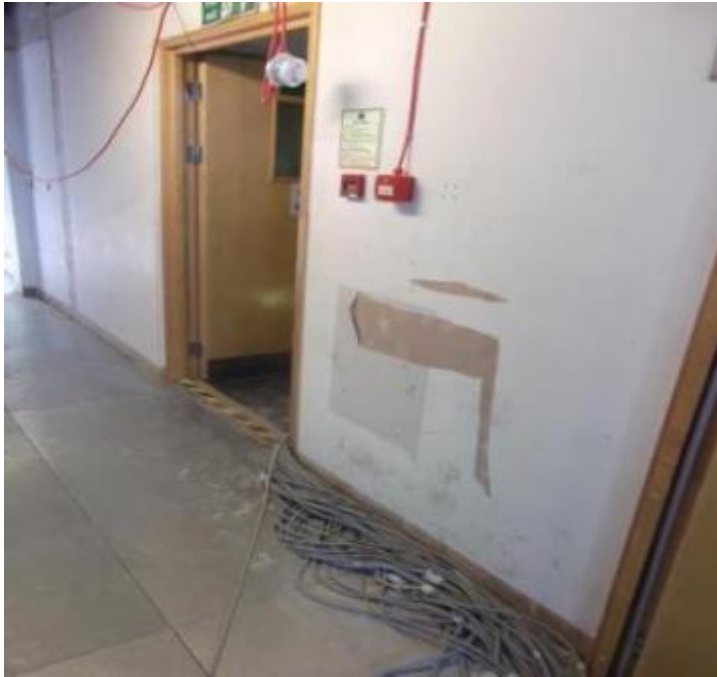
Figure 18: Unsecured electrical cables during refurbishment – photograph courtesy of Robert Bacon
