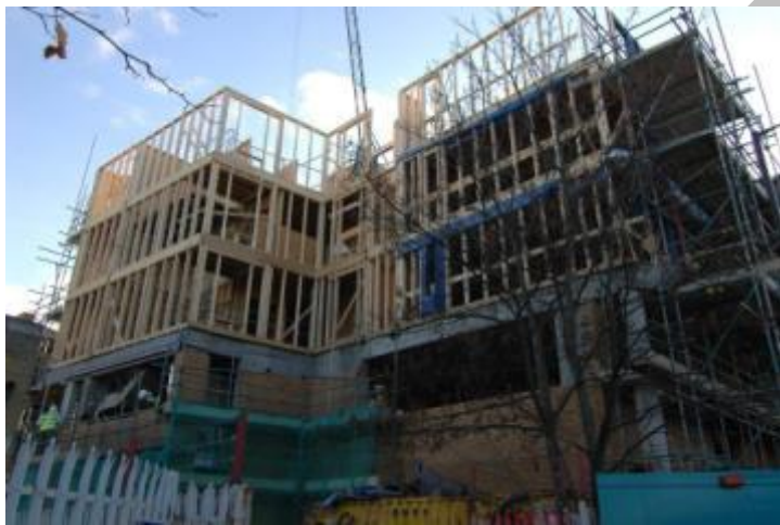
Figure 7: Timber frame extension on a traditionally constructed building – photograph courtesy of the Building Research Establishment
