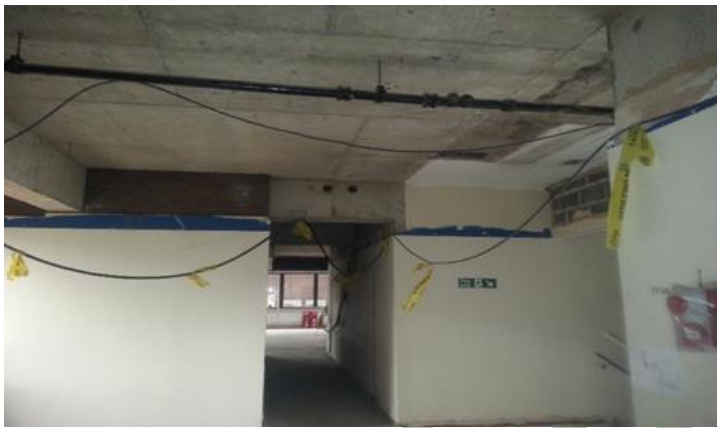
Figure 17: Live cabling during construction phase should be labelled; labelling may be destroyed by fire – photography courtesy of Nick Lacey
