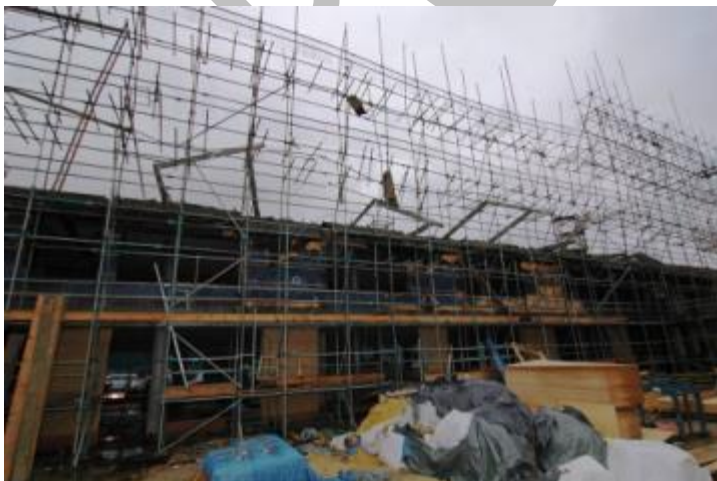
Figure 8: The same building following a fire in the timber frame extension – photograph courtesy of the Building Research Establishment
