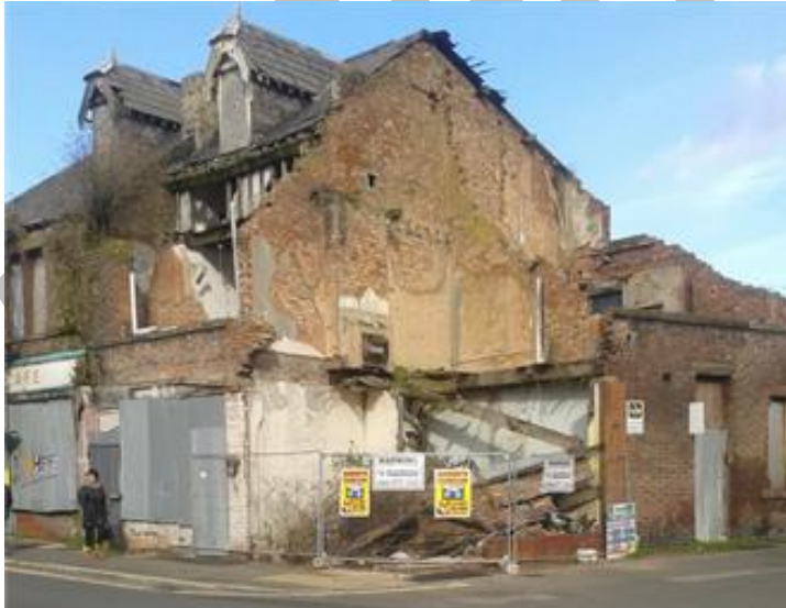
Figure 10: Derelict building – photograph courtesy of G. Pottenger
