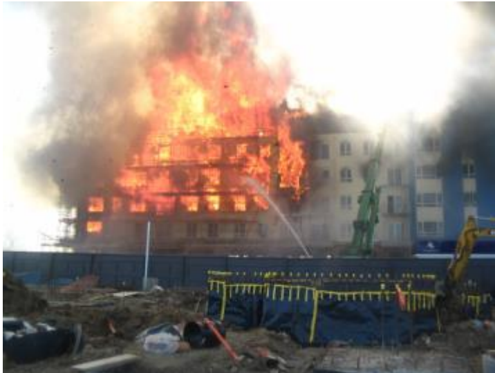
Figure 5: Timber building under construction at Colindale, London – photograph courtesy of London Fire Brigade
