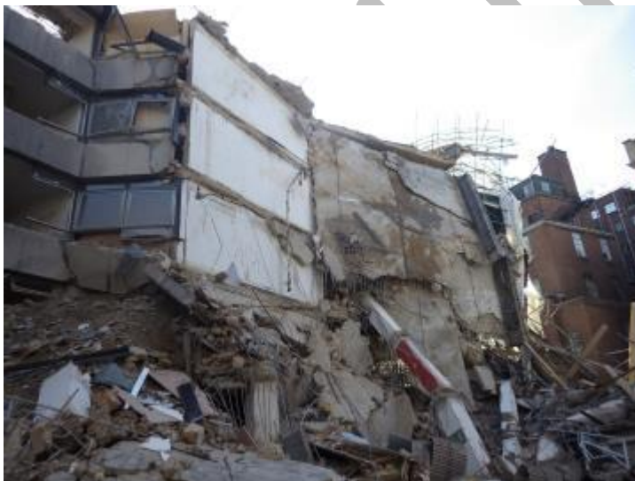
Figure 12: Building collapse during demolition at a site in Aldwych, London – photograph courtesy of London Fire Brigade
