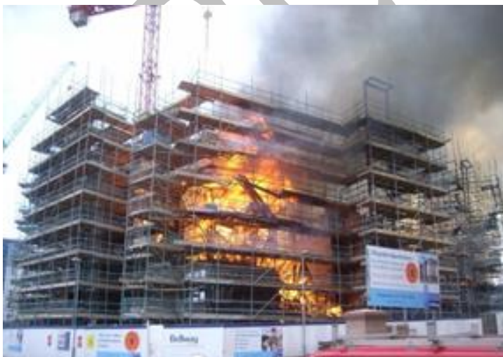
Figure 5: Building construction showing hoarding as a site boundary – photograph courtesy of John Dickie
