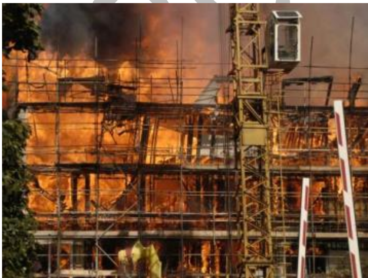
Figure 4: Fire in timber building under construction – photograph courtesy of London Fire Brigade
