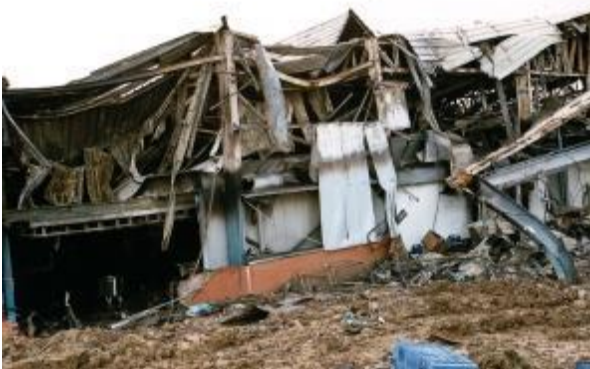
Figure 3: Structural collapse of building Source: Building Research Establishment
