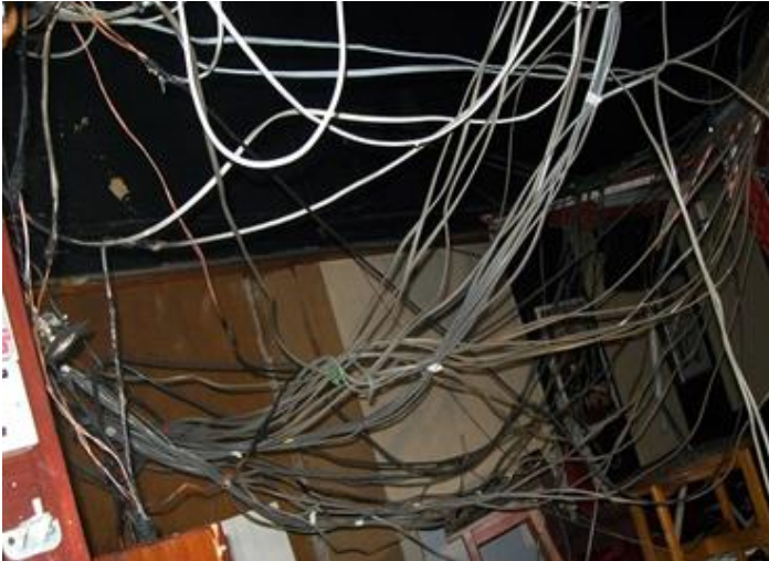
Figure 2: Cables dislodged from suspended ceiling fixings following a fire in compartment Source: B. Massie, Merseyside Fire and Rescue Service
