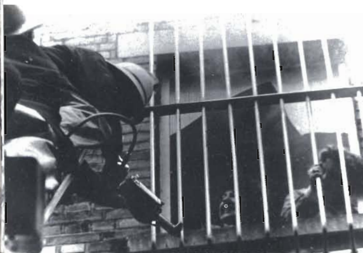
Plate 18. A mechanical saw being used to remove bars from a window at a large departmental store. Several women were rescued after being cut off by the fire.
