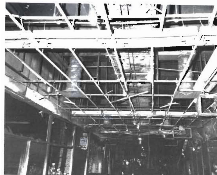
Plate 3. Part of the same precinct (see Plate 2) after a large fire. Asbestos panels have fallen away exposing the suspended ceiling framework and mechanical ventilation trunking. This trunking was externally clad with expanded polystyrene insulation which promoted fire spread and evolved toxic fumes. Photo: Merseyside Fire Brigade
