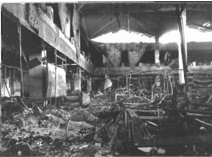
Plate 16. Covered market within a shopping precinct. In the foreground, left and hanging down from the roof, are panels of sprayed concrete on wire mesh. These became detached from their metal hangers and collapsed during the fire.
