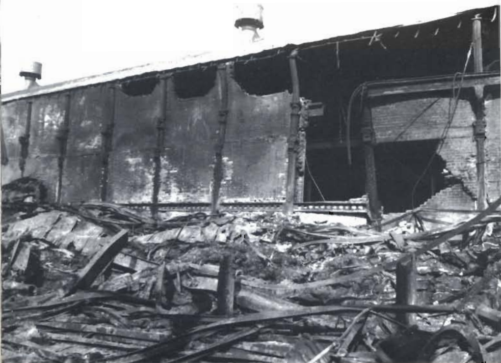
Plate 12 Various stages of collapse at a large fire in a general warehouse. Note the bent cast-iron columns in the back wall. Other cast-iron columns in the foreground have been snapped off short.
