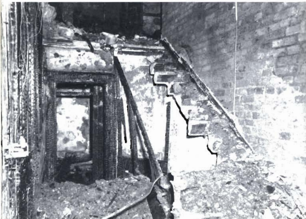
Plate 13 The effect of a severe fire on a stone staircase in a hotel. Photo London Fire Brigade
