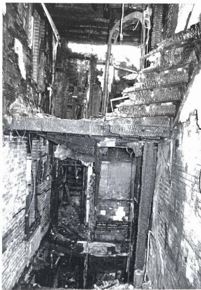
Plate 7 Remains of a hotel wooden central staircase. The disused small lift shaft (centre) acted as a flue causing almost complete destruction of the staircase and difficulty of access for the Brigade Photo East Sussex Fire Brigade
