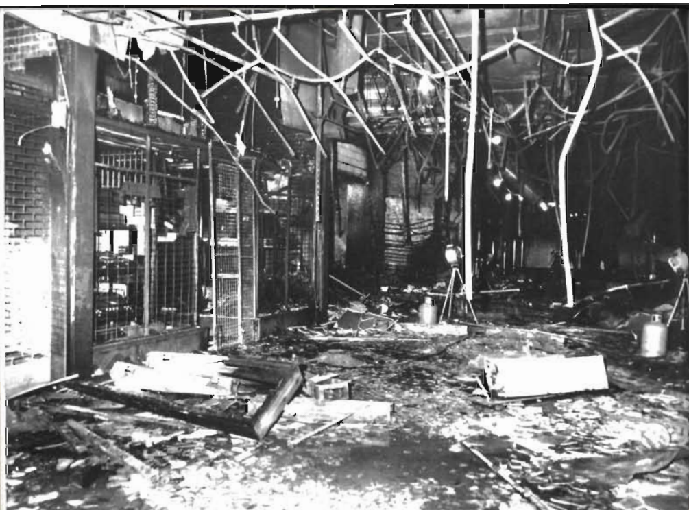
Plate 4 The intense fire in this shopping mall (see Plates 2 and 3) caused a general collapse of the suspended ceiling and mechanical trunking which hindered firefighting Photo Merseyside Fire Brigade
