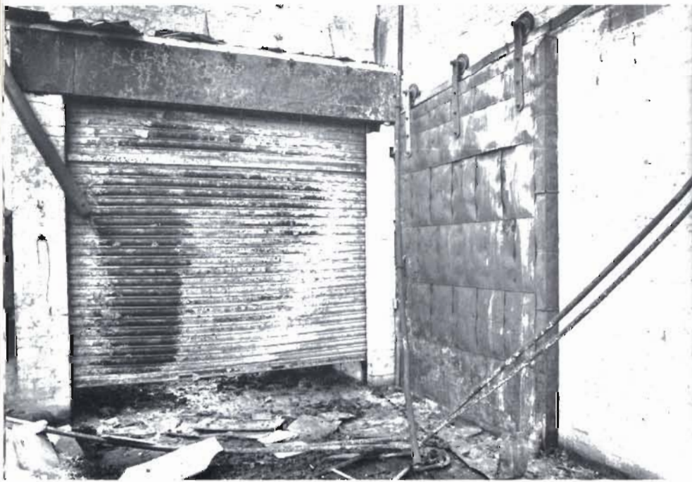
Plate 9. At this fire the fire-resisting sliding door on the right operated and effectively contained the fire. Unfortunately the sliding shutter, although operating successfully, jammed in the position shown allowing some spread. Photo: Bedfordshire Fire Service
