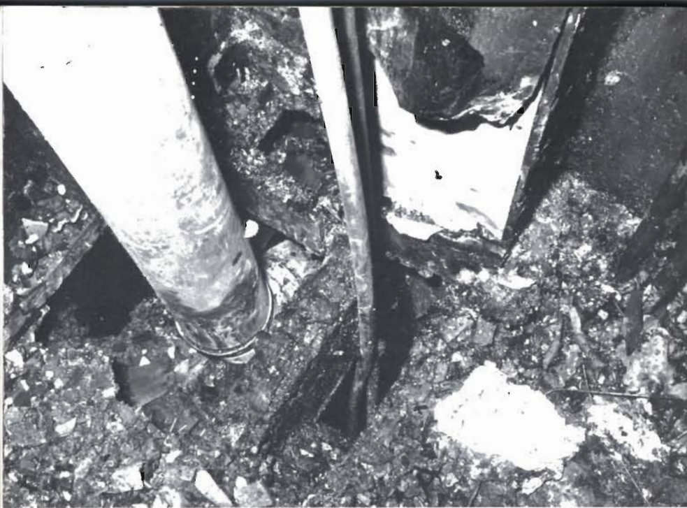
Plate 8. In this fire in a private house the central heating flue pipe was uninsulated throughout its entire length. There was no separation at all where it passed through the airing cupboard.
