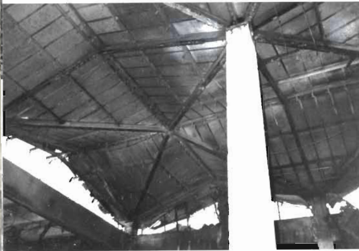
Plate 17 Example of modern light roof design. Wood wool panels covered externally by a layer of bituminous felt and copper cladding. The framework for them is of steel joists on reinforced concrete columns. The steelwork was protected by panels of sprayed concrete (see Plate 16) before their collapse.
