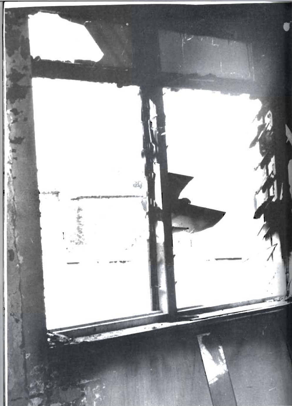
Plate 25 Evidence of illegal entry before a fire. Note the two unbroken louvre panes carefully removed and placed one under and one on the window sill. Photo Commissioner of Police, Gibraltar
