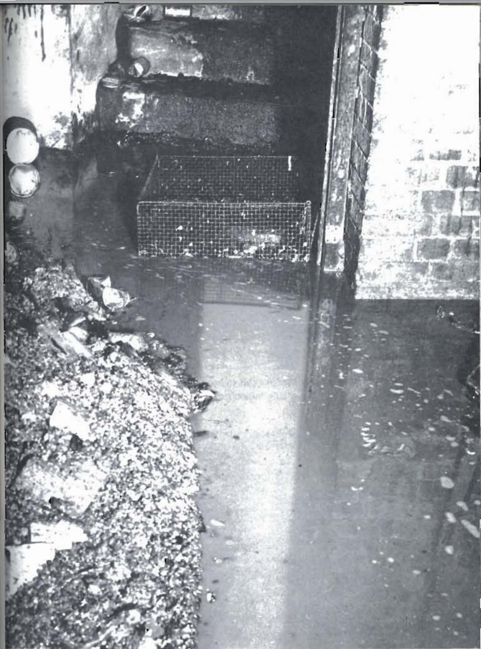
Plate 16 This wire mesh guard is protecting a drain from blockage by debris. Manholes should have similar protection Photo London Salvage Corps
