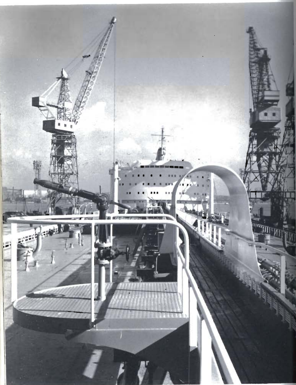
Plate S.17 Fixed firefighting monitors covering the deck of a tanker Photo. Stewart Bale Ltd.
