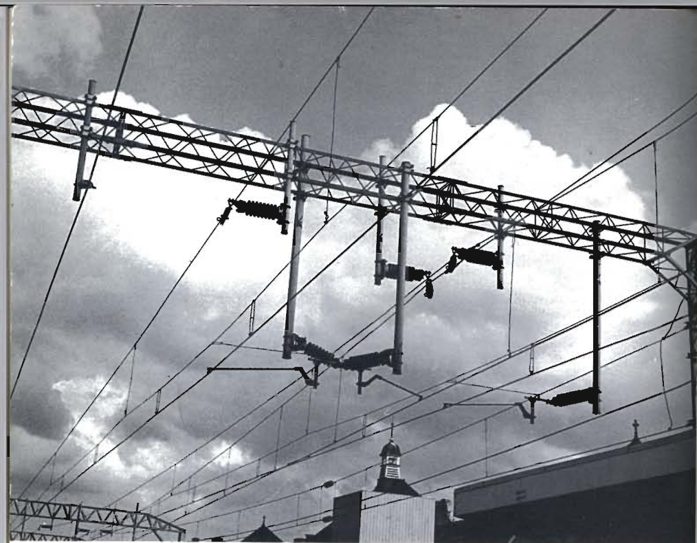
Plate R 3 Multiple overhead line equipment with 25 kv lines, tensioning devices etc Photo London Fire Brigade
