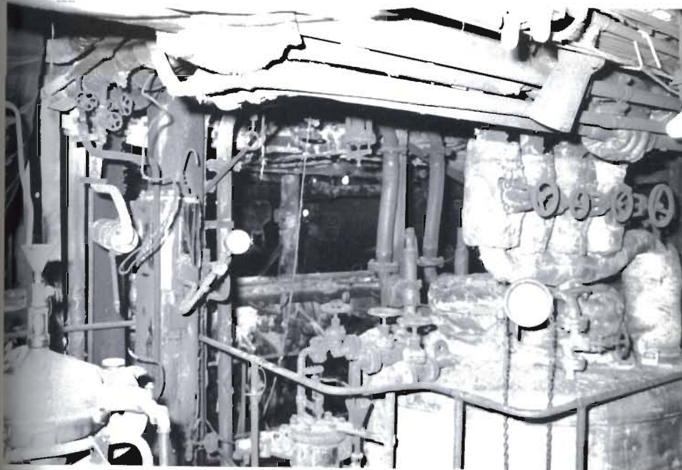
Plate S.19 The engine room of the car-ferry 'Norwave' following a fire. A horn nozzle of the CO 2 system can be seen above the valve group. The engine room was evacuated, the CO 2 system operated, and the ferry towed back into dock to enable the Brigade to tackle the fire. Photo. Humberside Fire Brigade
