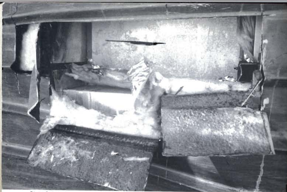
Plate R 9 An illustration of cutting into the roof of a carriage, showing the insulation, parts of the carlines, trunking and the ceiling of the compartment
