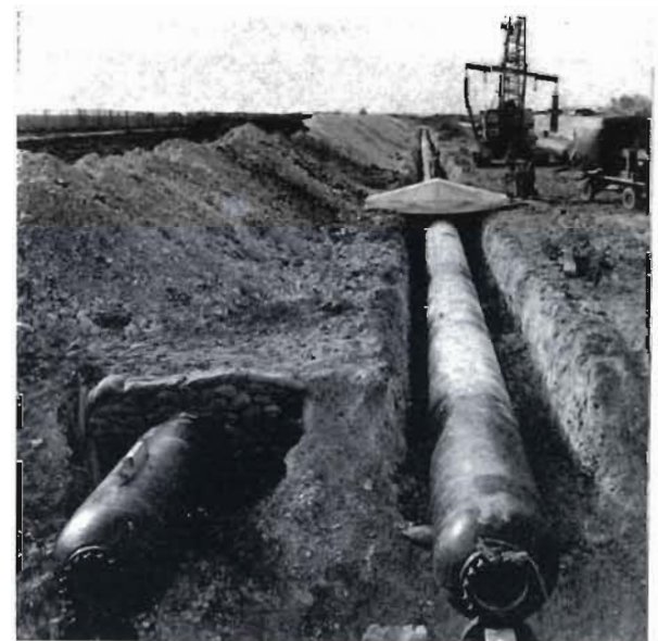
Plate 38. Underground high-pressure gas storage pipe clusters in the course of construction. These can be up to 500 ft. (152 m) in length.
