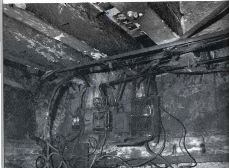
Plate 60. An example of an untidy domestic electricity installation which leads to a high fire risk. Arcing has occurred on the side of the larger fuse box and elsewhere.
