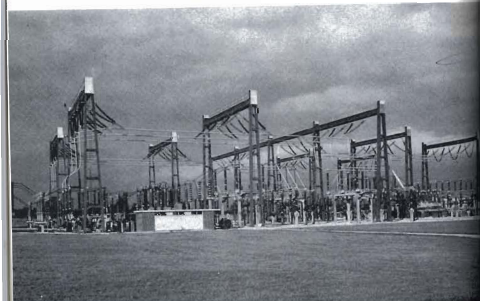
Plate 52. Part of an outdoor 275/400 kV substation showing how the connecting conductors are kept well above ground level.
