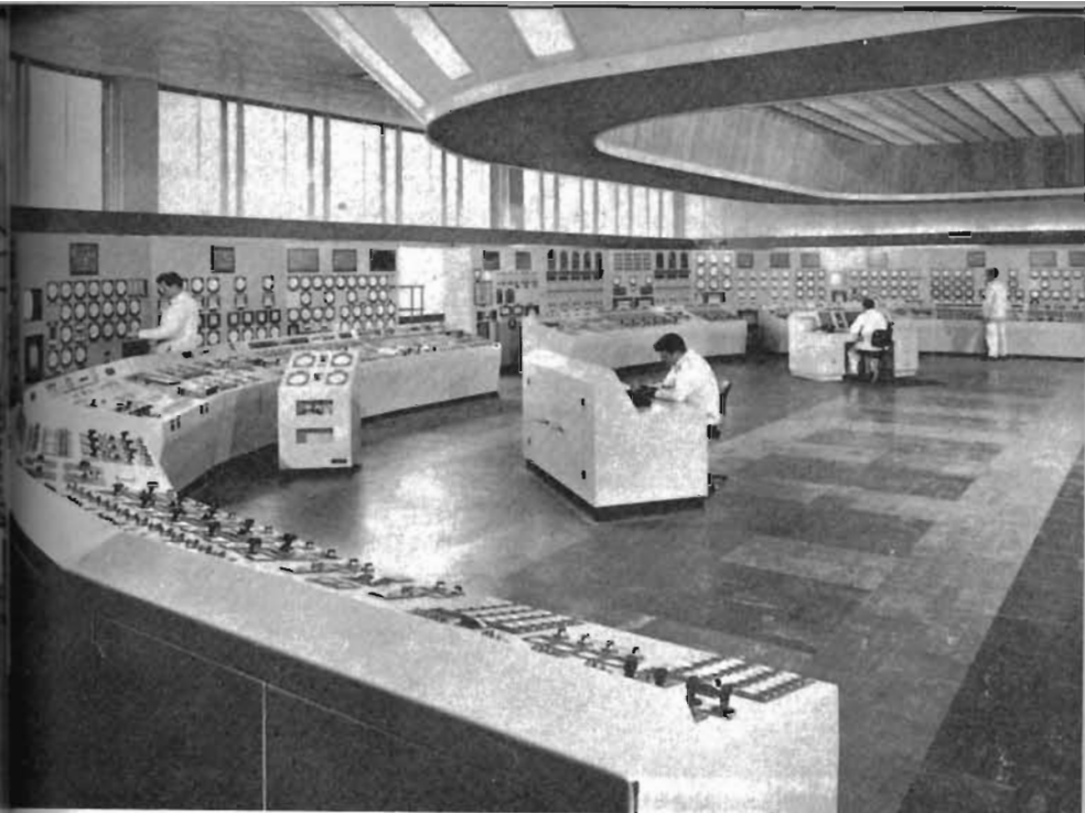
Plate 57. Part of the main control room at Ferrybridge power station. All the boiler/turbine units together with auxiliary plant and gas turbines are controlled from this central control room. The 2,000 MW output is fed into the national grid by three double circuit 275 kV overhead lines.
