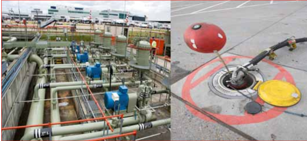
Picture 18 and 19: Fuel farm pump raft and apron fuel hydrant
