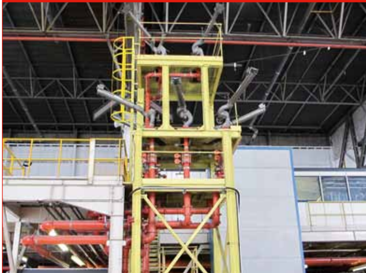
Picture 16: Fixed installation foam tower which forms part of a foam fire suppression system in a large maintenance hanger
