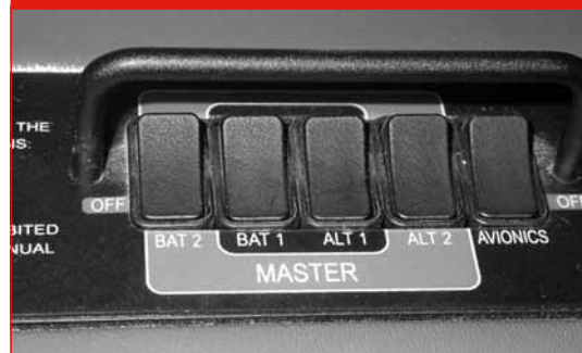
Picture 6: Master switch
