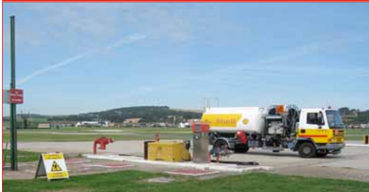
Picture 20: Fuelling station at Shoreham Airport
