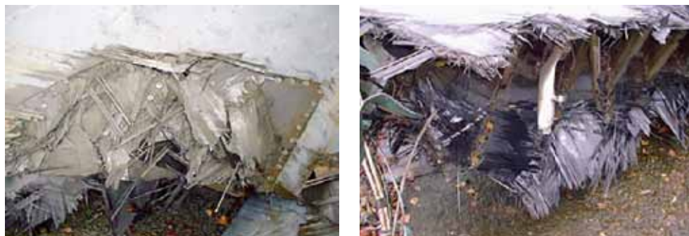
Pictures 3 and 4: Example of delaminated and exposed fibre post aircraft crash
