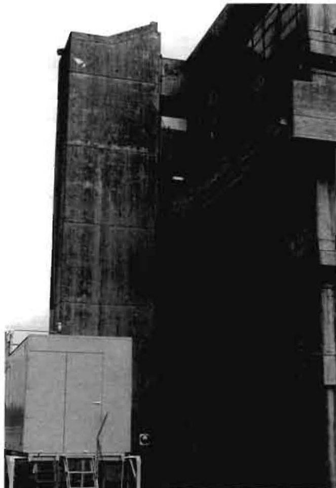
Figure 2 Industrial 'A' Building Showing the North Stairwell Entry Door and Landing Windows
